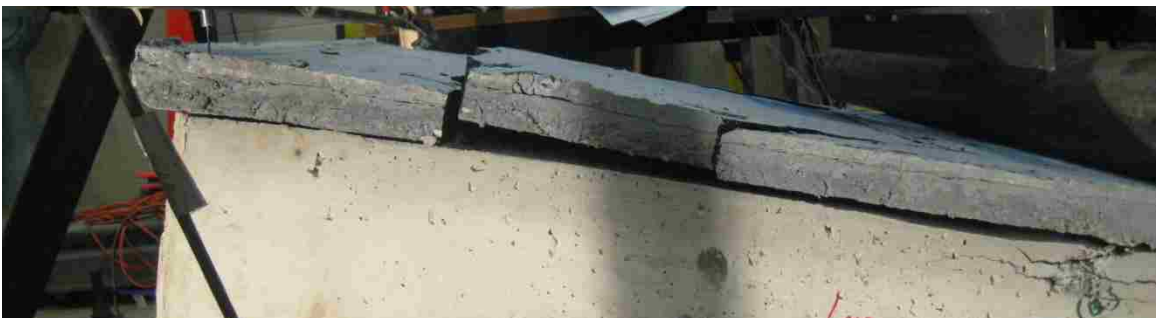
Figure 5.18: Horizontal shear failure of the UHPC outside of the shear- friction reinforcement (profile)
